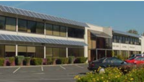
Solar panels installed by apprentices and Journey level electrician at the Puget Sound Electrical Joint Apprenticeship and Training Committee training center.
