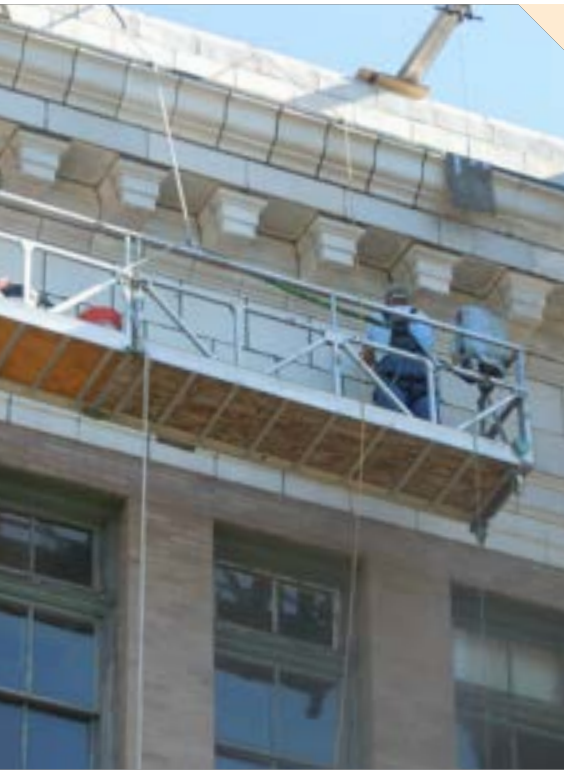
Bricklayers and Allied Craftworkers Local 1 members conducting a terra cotta building restoration on a Seattle public high school.
