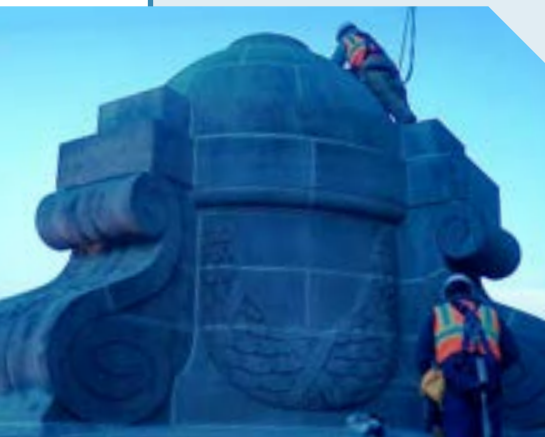
BAC Local 1 Washington members working on a restoration project at the State Capital.
