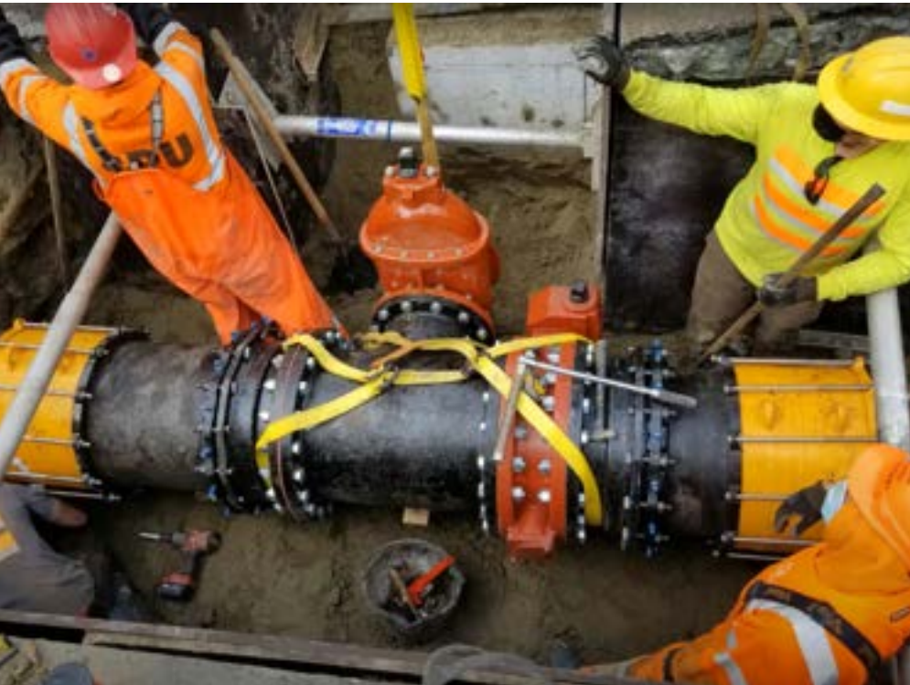
Plumbers and Pipefitters Local 32 water utility workers with Seattle Public Utilities installing a water main.
