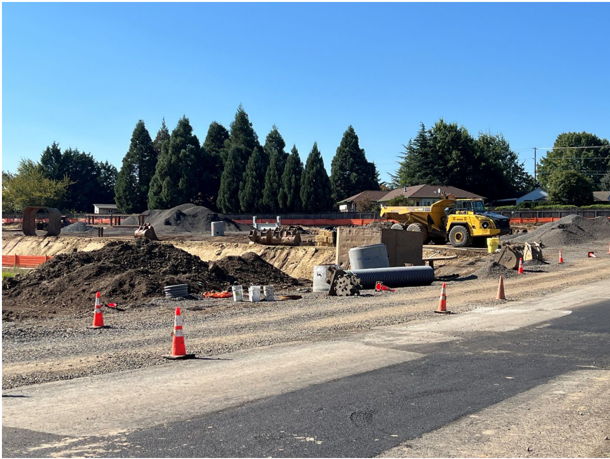
Active construction for Greely Farms Phase 2B and 2C subdivision. Photo taken October 6, 2024, from the subject property. The new Greely Pump Station will be in this development by the street.
